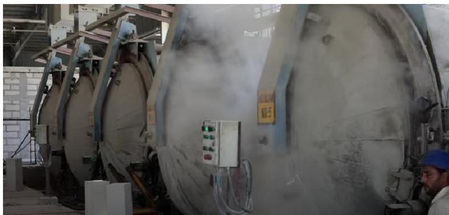
Steam Curing Process (Autoclave Reactor)
